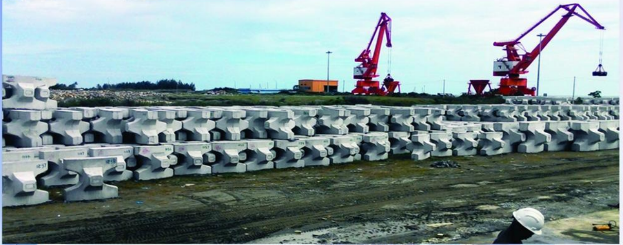
Breakwater Improvement Project - Material Armor Block - Location of Suak Puntong Village, Nagan Raya District, Nangroe Aceh Darussalam
